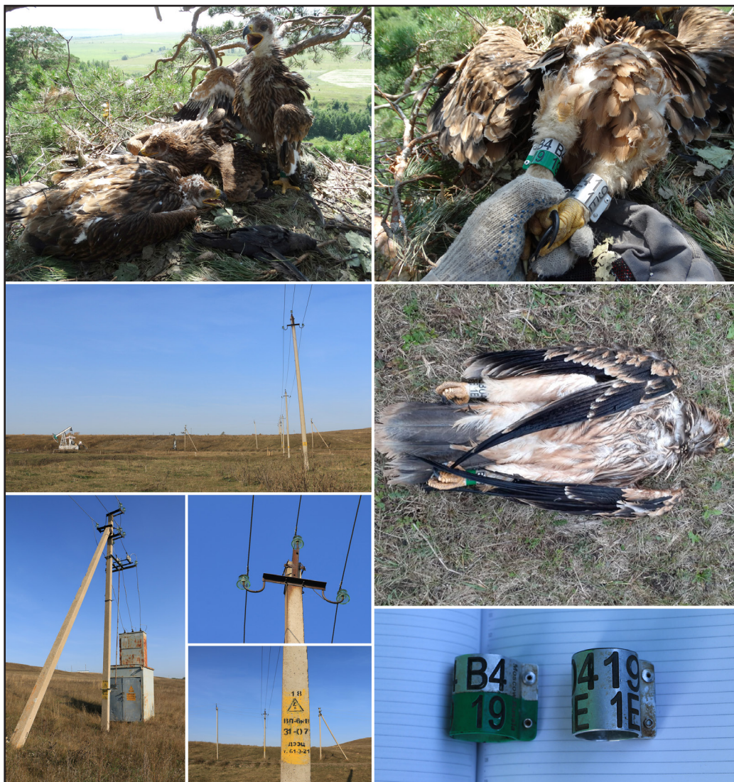
Fig. 2. Power line 6 kV dangerous for birds on the outskirts of the village of Novaya Kashirovka in Almeteyevsky District at the site of the death of an Imperial Eagle fledgling in September 2020 (bottom at the left). The eagle's corpse on the day it was found under a power line and rings (AB-0419-1E and B-419) removed from the eagle's corpse (bottom at the right). This was one of three nestlings tagged in the nest on July 8, 2020 (upper). Photos by R. Bekmansurov.
